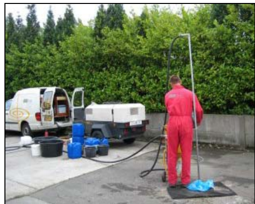
Figure 6. Injection of carbon source and nutrients between Pb4 and Pb8 in progress
