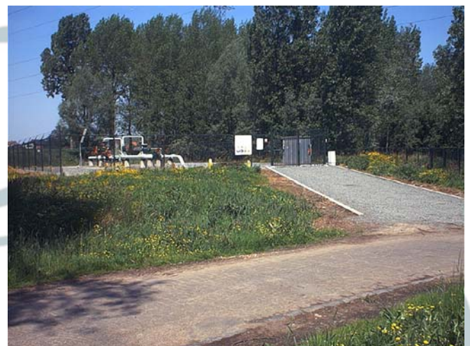
Line valve station Pu at Bornem/Hingene
