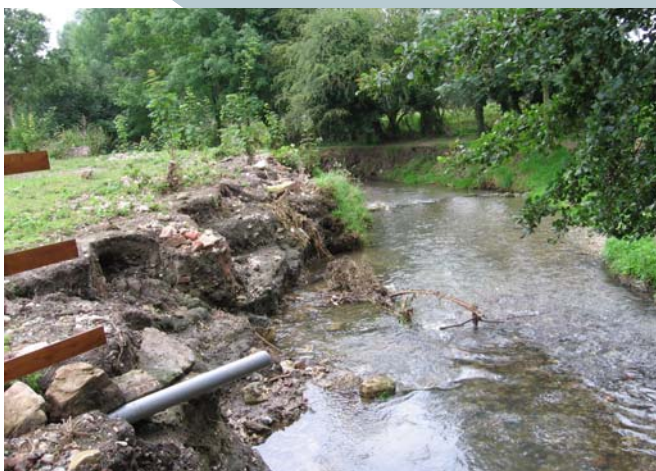
Damage after a flood
