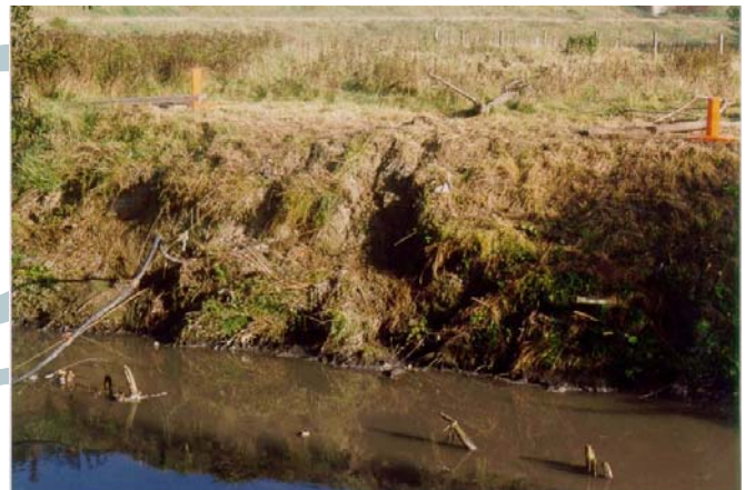
Riverbank erosion (situation before works)
